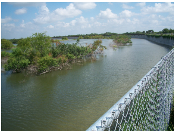
Pictured: Bentsen-Rio Grande Valley State Park, which is near the Rio Grande in mission, TX, shortly after Hurricane Alex in 2010. The flood walls kept the water from spilling over into an RV retirement village on the other side.
