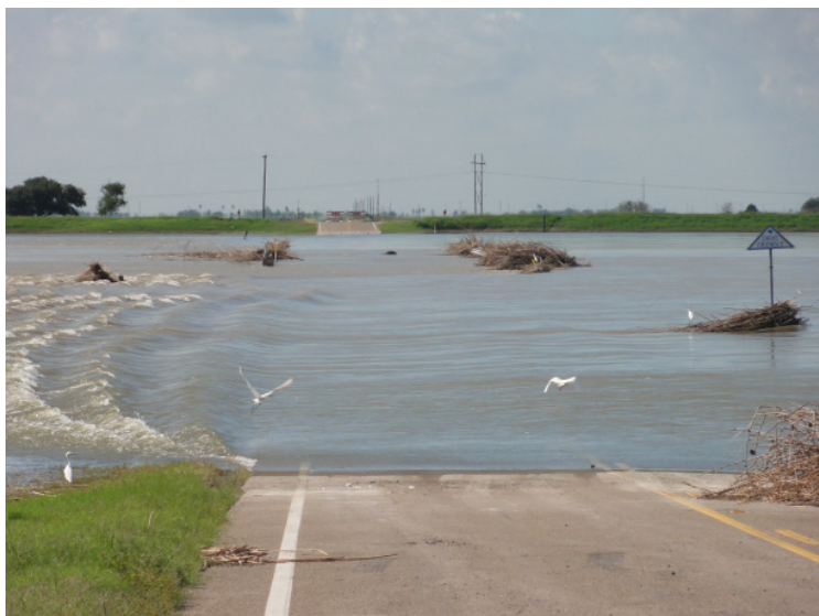
Pictured: Major highway in the Lower Rio Grande Valley near McAllen, TX, shortly after Hurricane Alex in 2010.
