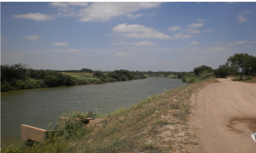
Pictured on left: CRP Station 13177, Rio Grande at El Jardin Pump Station
