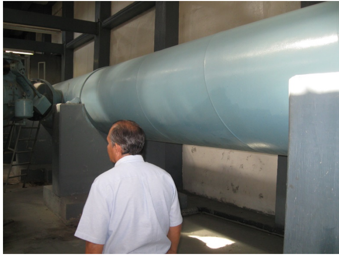
Discharge through a 60" diameter force main.
