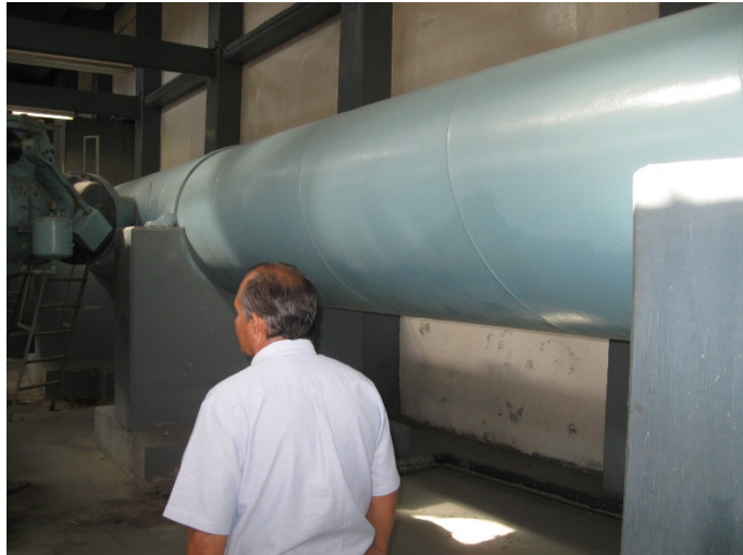
Discharge through a 60" diameter force main.
