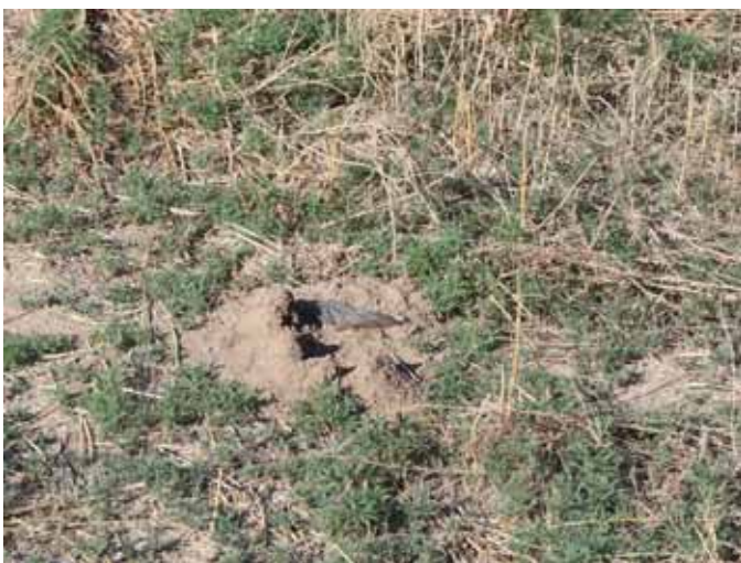
Gopher holes on south river side levee slope.
