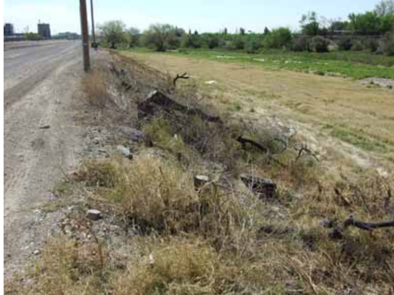
Downstream view of levee with dry, fallen trees and dry brush and grasses.
