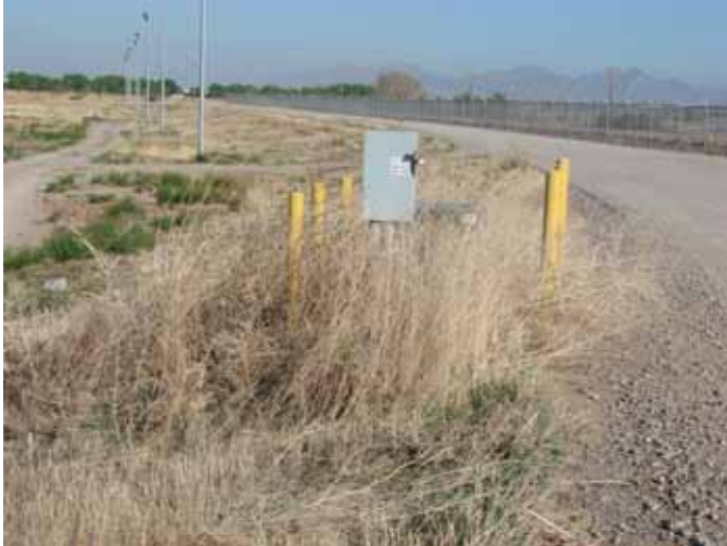
Border Patrol electric boxes on levee slope
