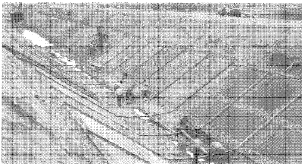
Plate 9. Open Section "A" Showing Configuration of Construction Joints and Gravel Drains Common in All Open Sections, 31 December 1937.
